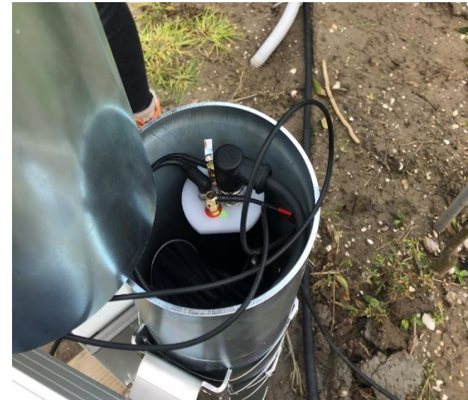
Data collection and transmission modem
